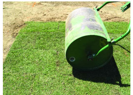
Figure 5. Rolling eliminates irregularities and establishes good contact between the sod and soil.
