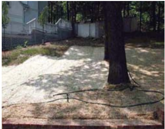
Figure 4. Various erosion control blankets can be used on slopes to help reduce erosion and retain soil moisture during establishment.
